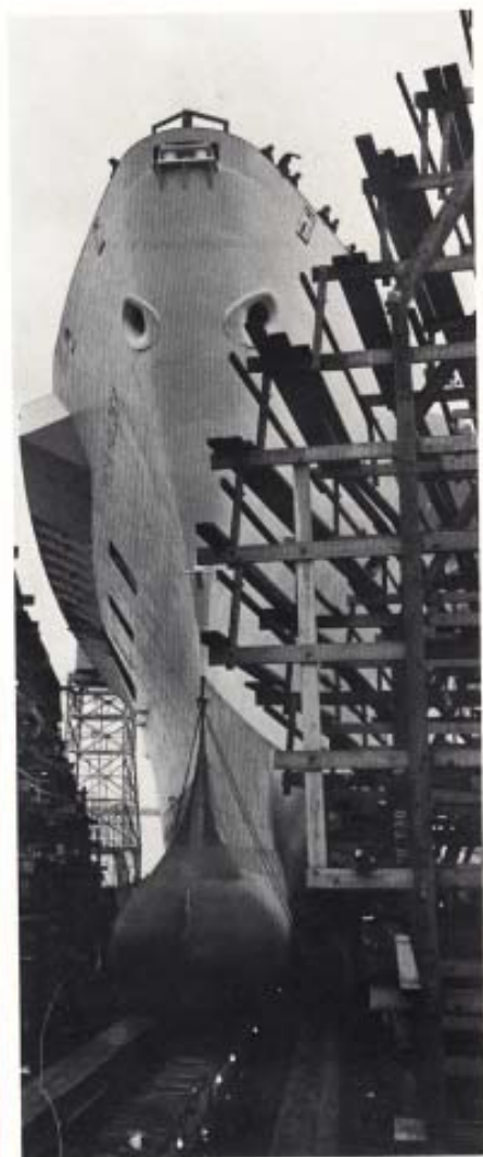
TRANSAMERICAN TRAILER TRANSPORT's new SS Eric K. Holzer launching at Sun Shipbuilding and Dry Dock Company, Chester, Pennsylvania November 11, 1970.
