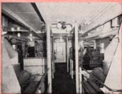
Looking forward, upper engine room, showing main engine exhaust manifold, two auxiliary generators, ship's service switchboard.
