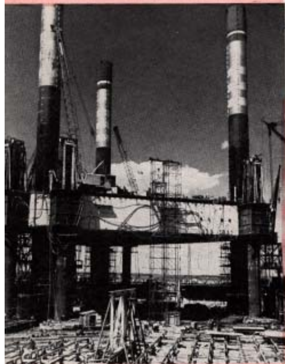
Closeup view of tower during latter stages of construction, in the building ways, South Portland.
